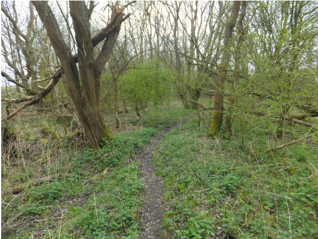
Figure 6 Looking south along the trackbed between Charwelton and Woodford Halse where the overgrowth is thicker than the section further north (roughly SP 5435 5466).
