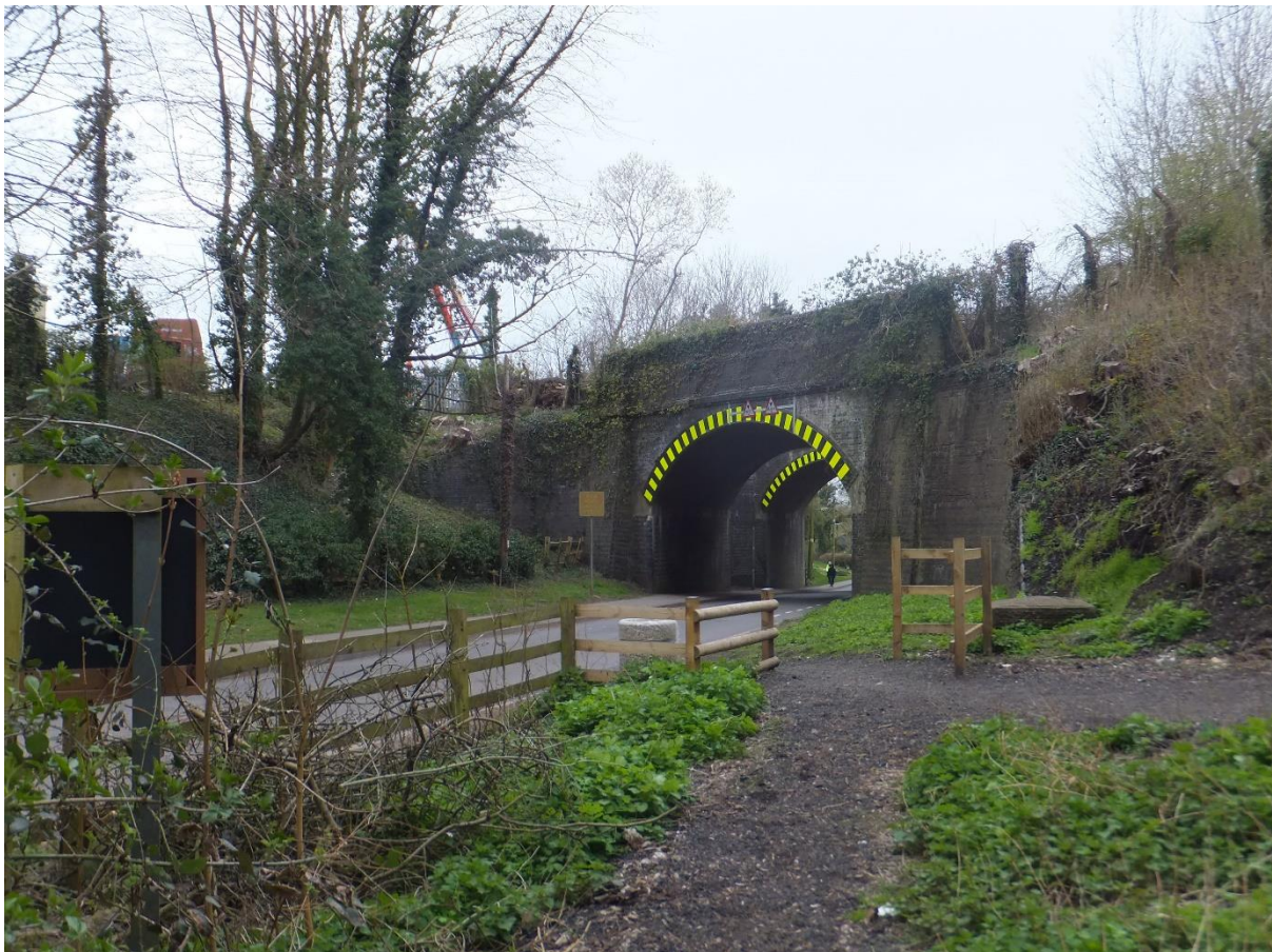
Figure 1 Looking south-west along Station Road in Woodford Halse at the bridges that would have carried the GCR (camera at SP 5406 5257).
