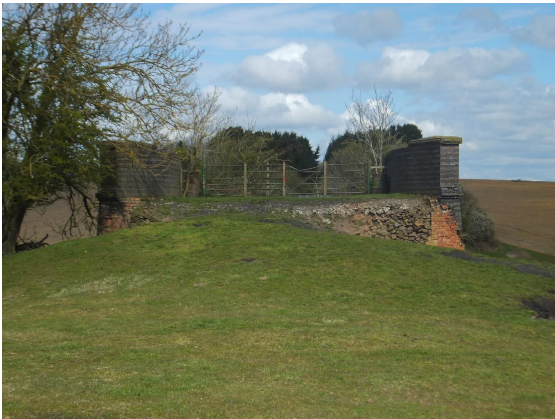
Figure 6 A view north towards the blocked southern end of the Catesby Viaduct (SP 5215 6046).
