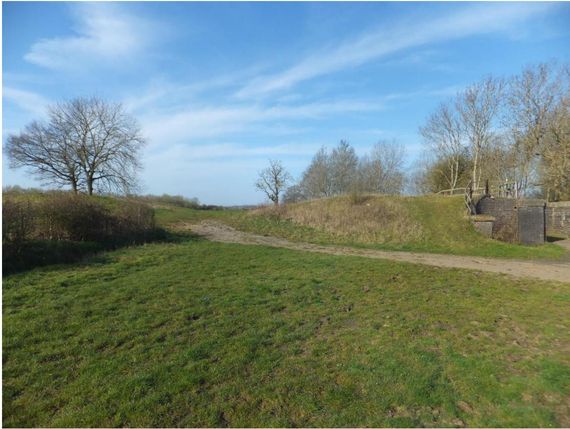
Figure 13 Looking west just south of the missing bridge at SP 5185 7089, showing how the embankment has been partly demolished.
