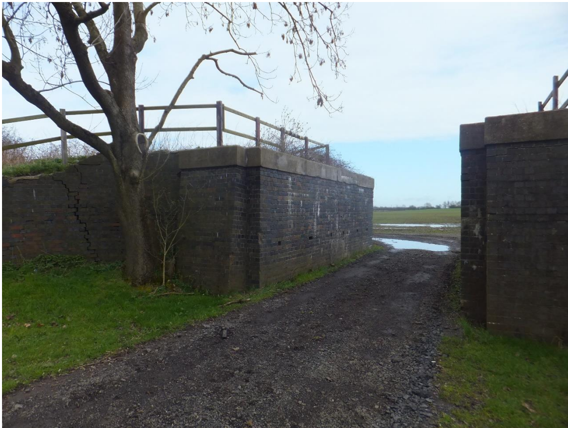
Figure 14 Looking east at the missing bridge (SP 5185 7089).
