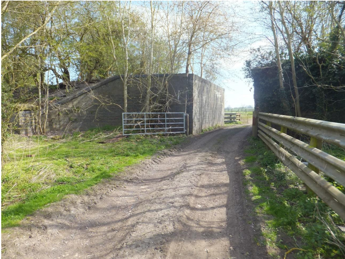
Figure 2 Looking east at the gap in the embankment near the A45 at Willoughby (SP 5239 6744).
